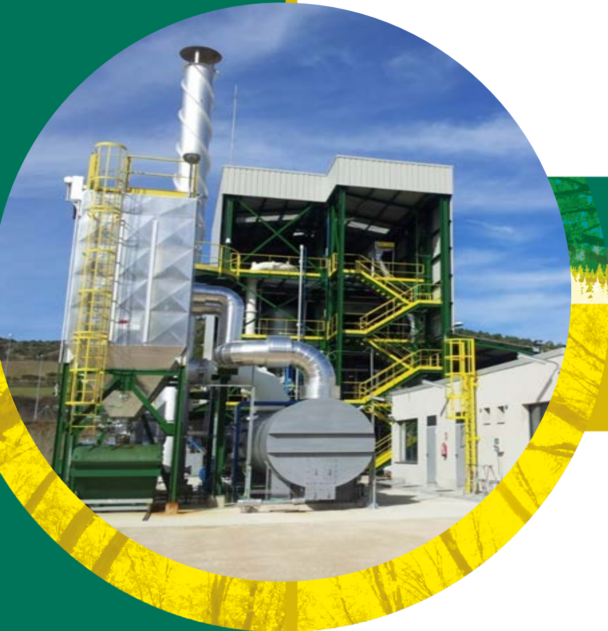
CENER biomass gasification plant, Aoiz (Spain)
