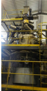
Figure 1: NOTAR® Gasifier on P11
