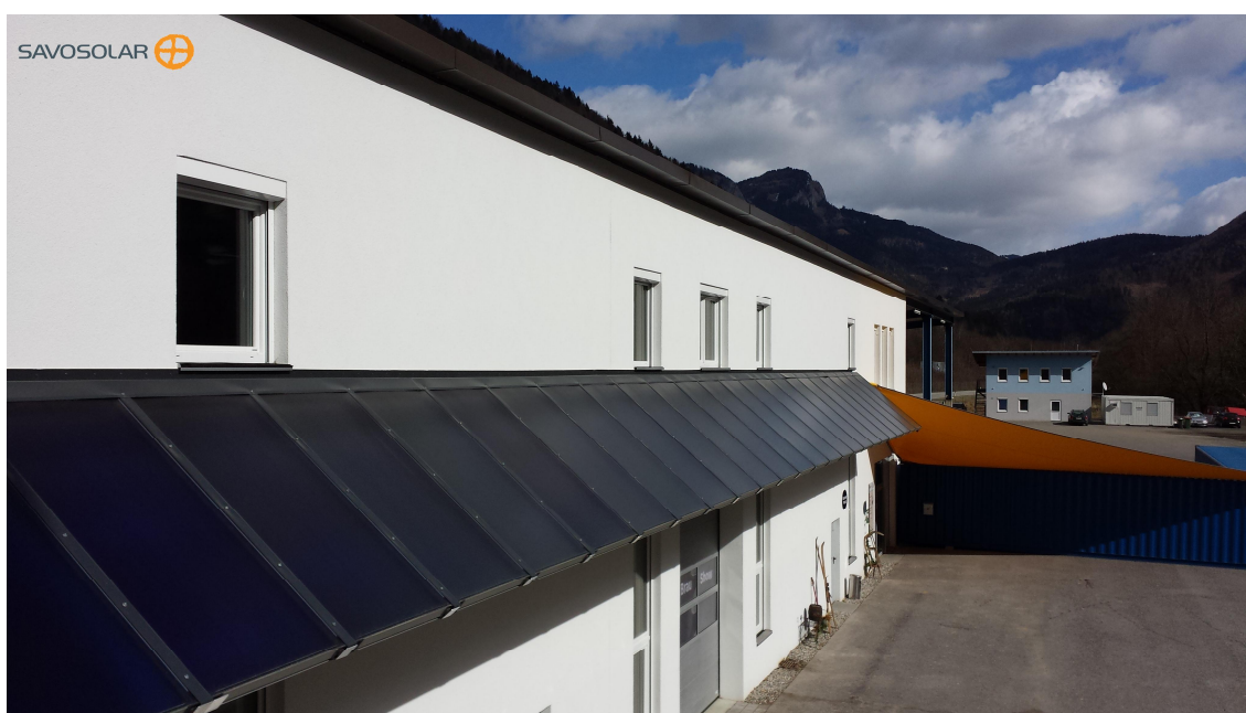
Figure 14. Savosolar's collectors for process heat production in a brewery in Austria, ©Savosolar.
