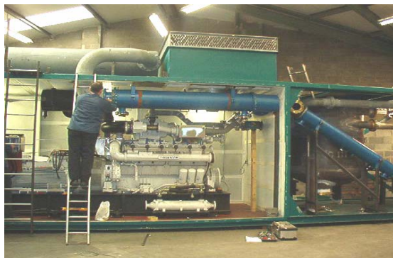
Figure 33: Exus Energy 300kWe module.
