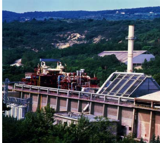
Figure 19: TPS CFB BMG Plant in Greve, Chianti (2x15 MWth Gasifiers)
