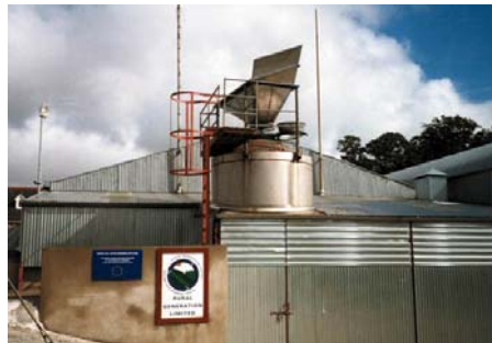
Figure 31: Brook Hall Estate Gasifier (Capacity: 100KWe)
