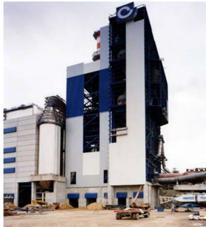
Figure 15: Lurgi Waste Gasification Plant in Rüdersdorf
