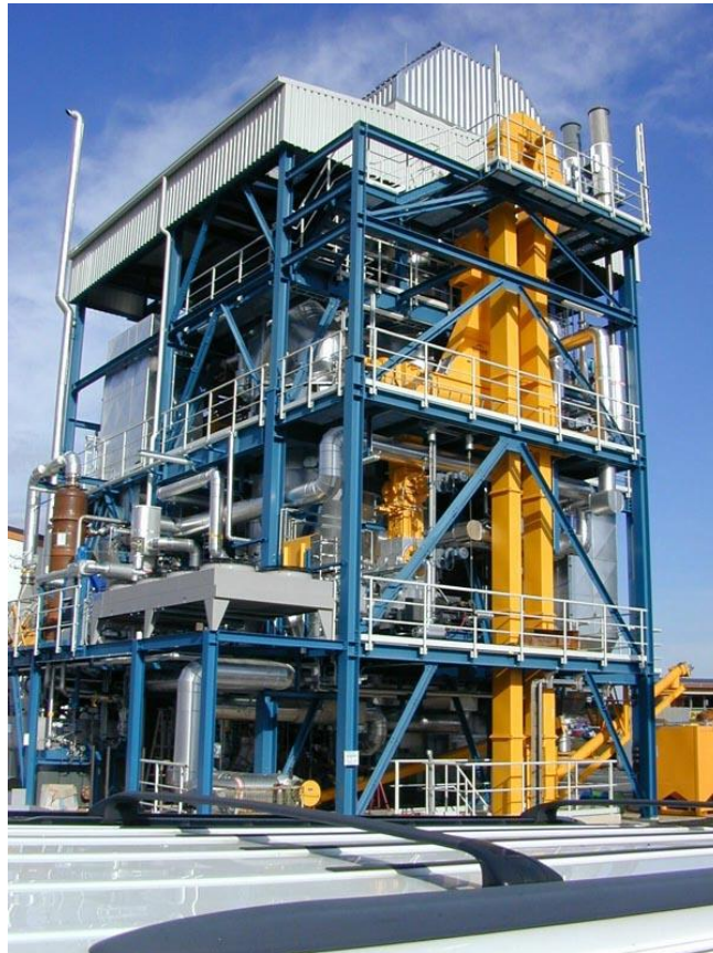
Figure 1: FICFB gasifier in Guessing
