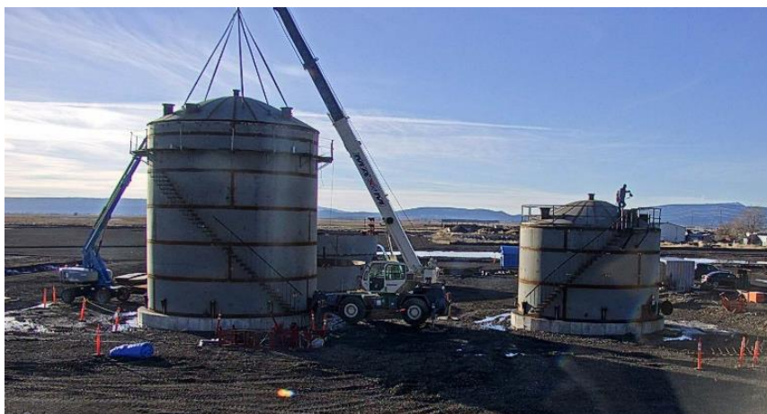
Figure 83: Construction progress, Red Rock Biofuels Lakeview facility (Source: 2019 DOE BETO Project Peer Review Update 5 March 2019)
