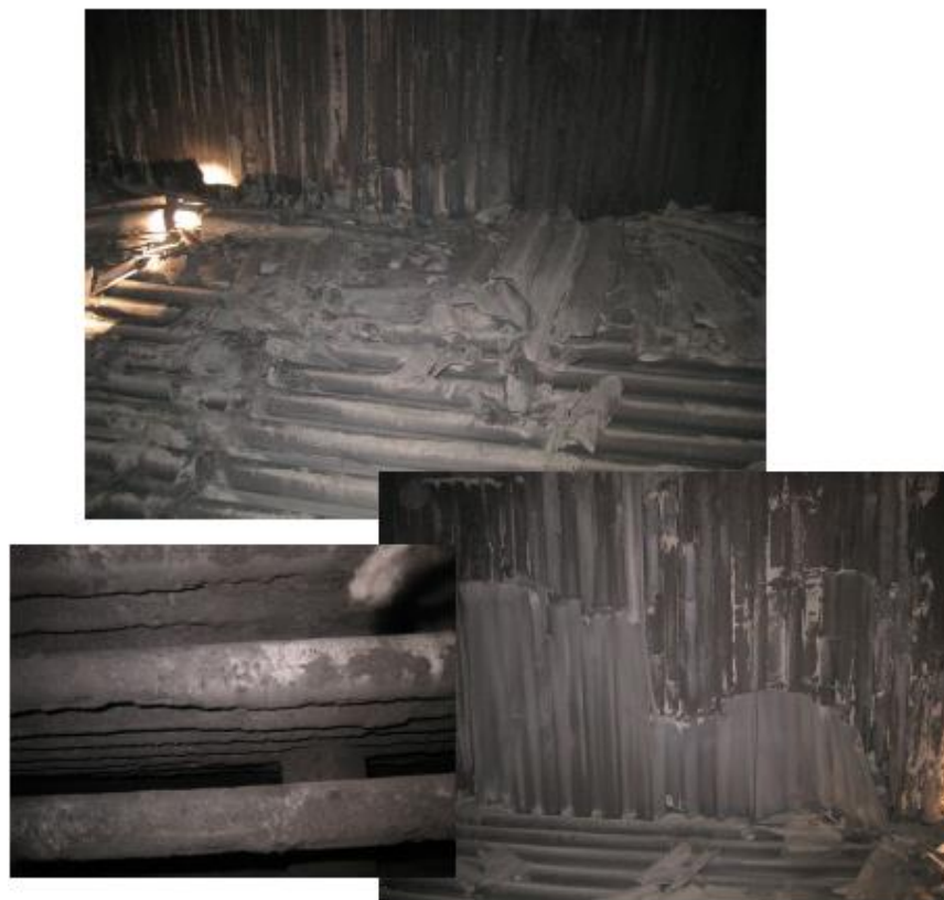
Figure 53 Amergas gas cooler 271 .
