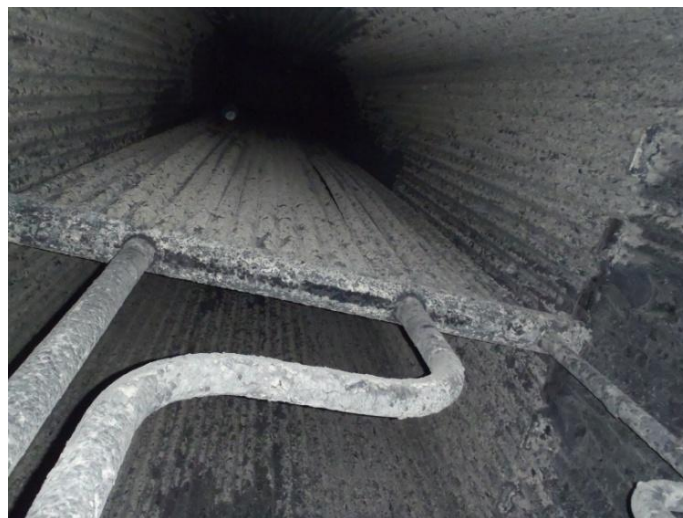
Figure 73 A photo of the gas cooler in the Kymijärvi II plant 389
